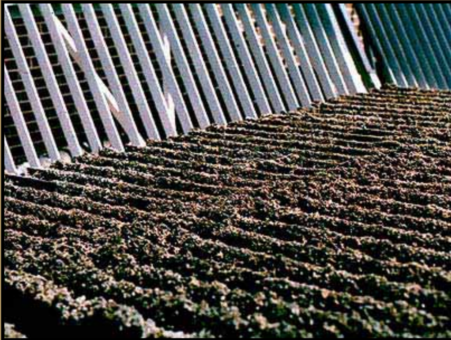
Fouled Trash Rack, Corps of Engineers
