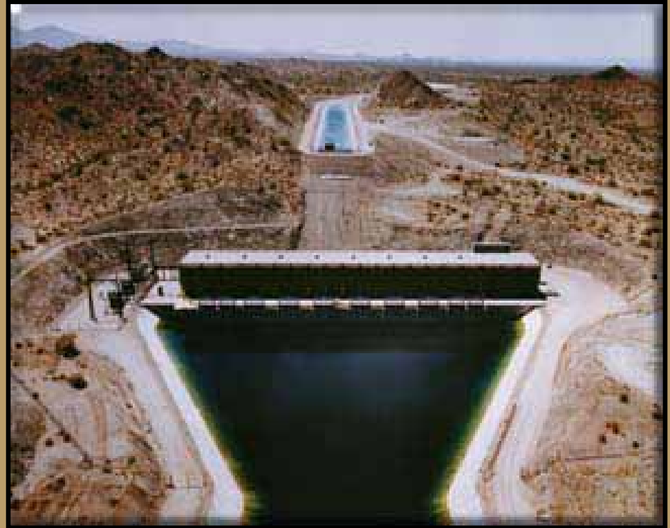
Bouse Hills Pumping Plant, CAP
