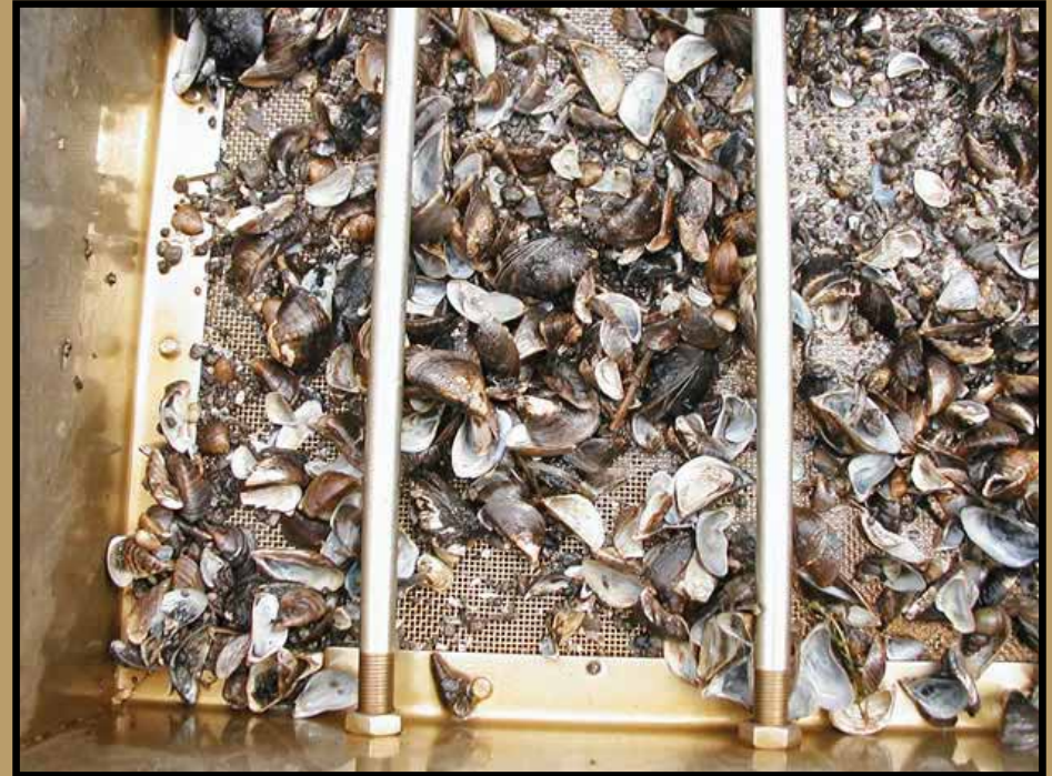
Intake screen blocked by shells
