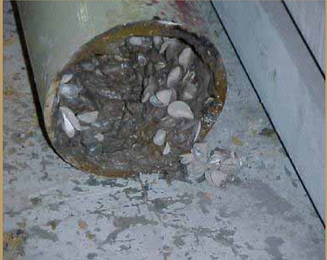
Water Cooled Transformer Piping
