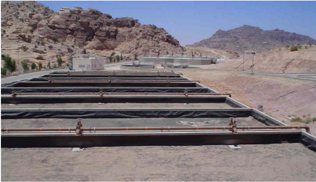
Figure 4. Conventional Sand Drying Beds at the Wadi Mousa WWTP.
