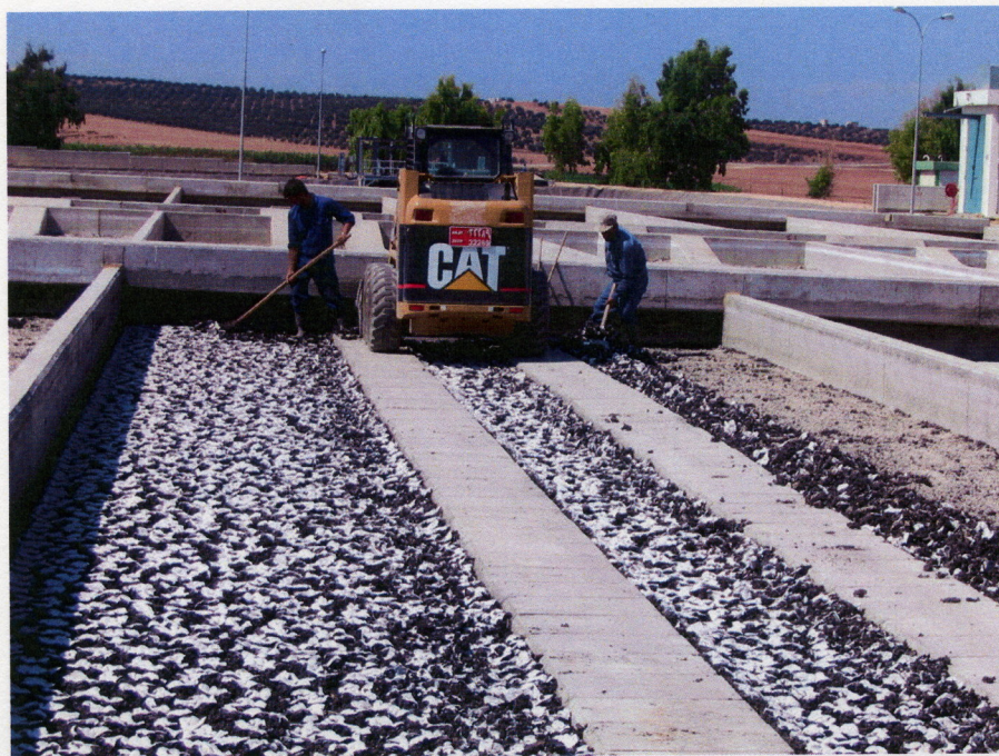
Figure (23): Dewatered sludge disposal at Ramtha treatment plant.
