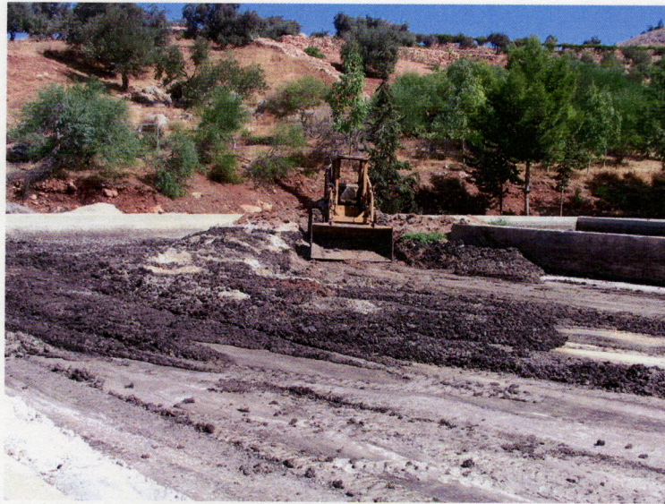
Figure (27): Dewatered sludge disposal at Kufranjeh treatment plant.
