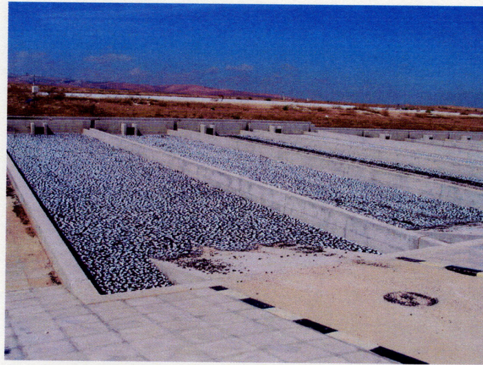
Figure (20): Drying beds at Wadi Hassan treatment plant.
