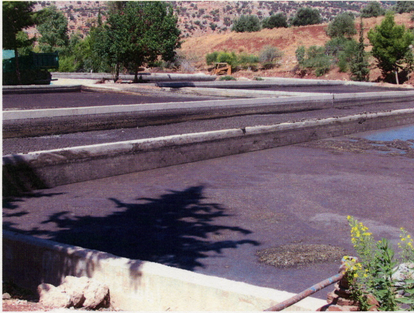
Figure (25):Drying beds at Jerash treatment plant
