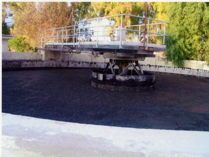
Figure (17): Sludge thickener at Central Irbid treatment plant.
