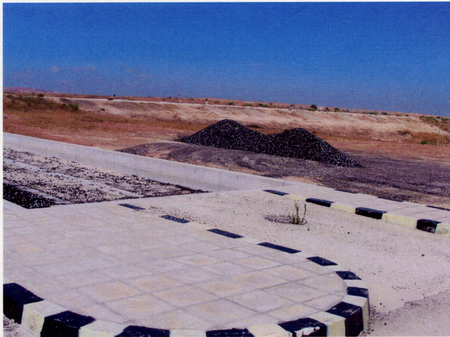
Figure (21): Sludge accumulation before disposal at Wadi Hassan treatment plant.
