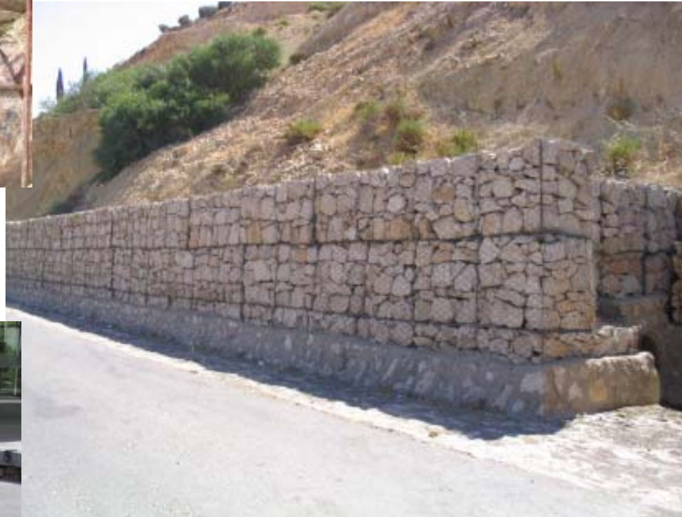
Gabions as they are traditionally used for soil stabilization along a roadway in Jordan.
