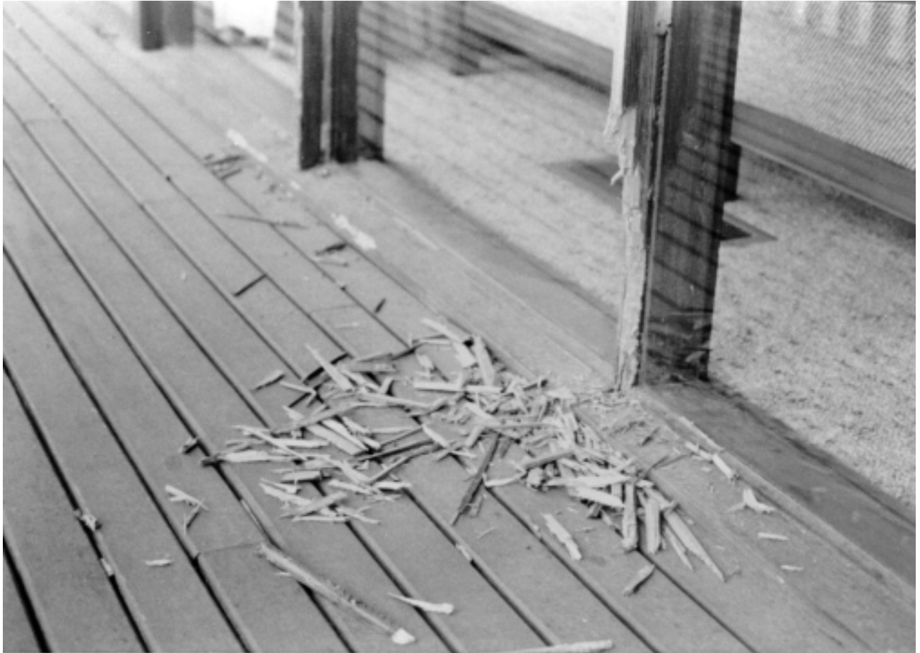
Figure 2 Damage to window frame by Sulphur-crested Cockatoo Photograph: I. Temby
